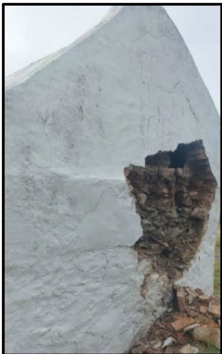
Collapsed Wall of the Livingstone Cottage
